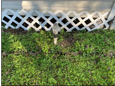
No natural gas meter installed at left side exterior
