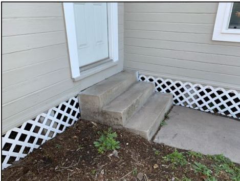
Back exterior steps not level/No handrail installed
