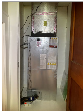
Trane HVAC equipment
