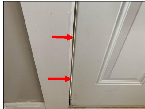
Back exterior door failed to seal closed properly
