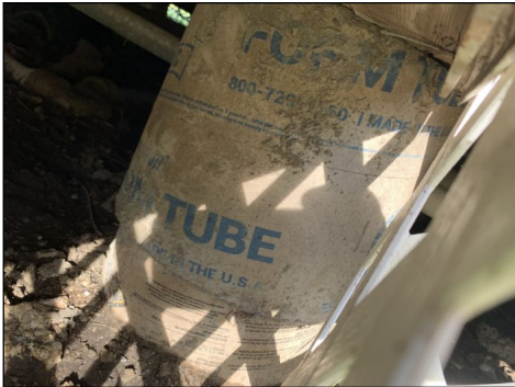
Paper/cardboard on foundation pier
