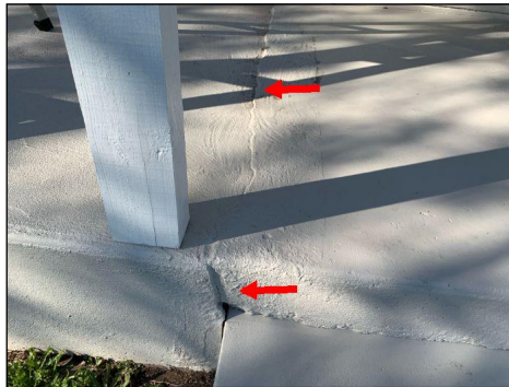
Front porch slab cracking
