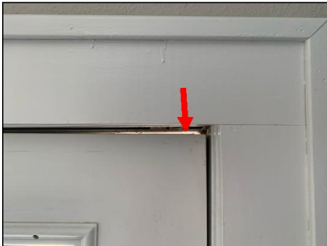
Front exterior door failed to seal closed properly
