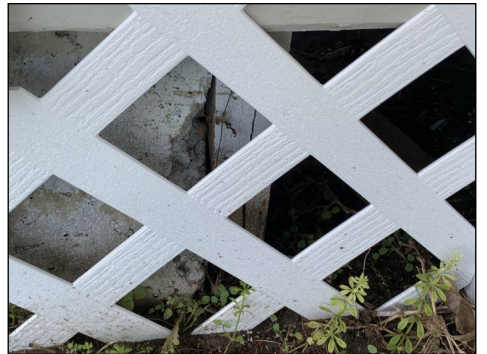
Damaged foundation pier/block
