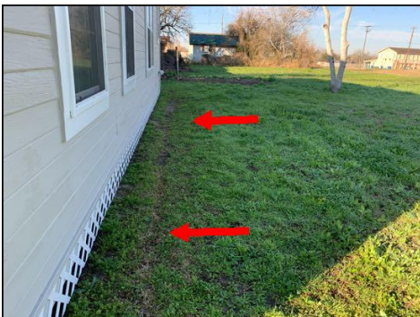
Grade slopes toward the crawlspace at the right side of the home
