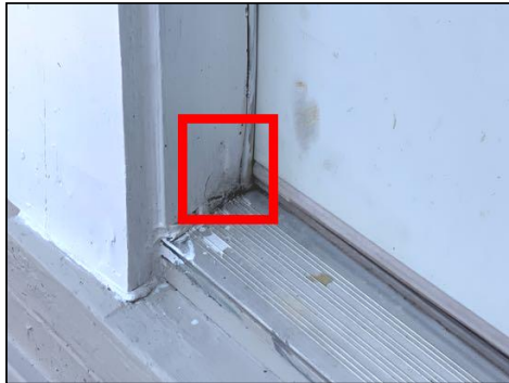
Wood trim decay/rot at the back of the home
