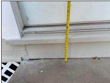
Top step to door threshold exceeded 7 3/4 inches in height
