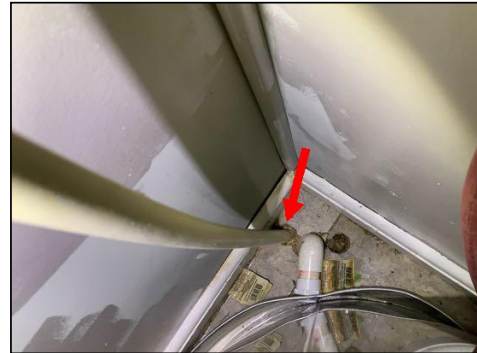
TPR valve discharge plumbed below the home
