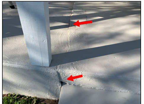
Front porch slab cracking
