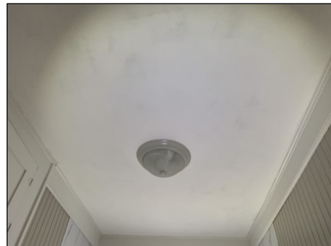
Black microbial growth on hall bathroom ceiling
