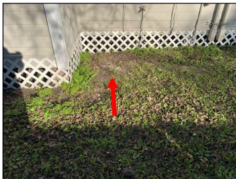
Grade slopes toward the crawlspace at the left side of the home
