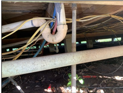
Drain plumbing leaking beneath the home/bathroom
