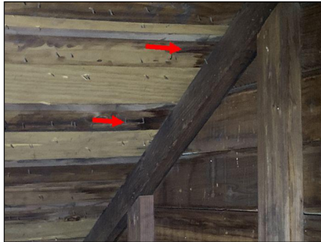
Moisture stains on roof structure in attic space
