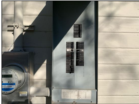
Main panel at left side exterior
