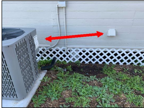
Dryer vent termination too close to back exterior condensing unit
