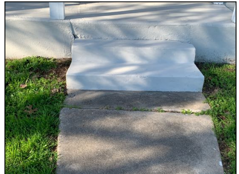
Front exterior steps not level
