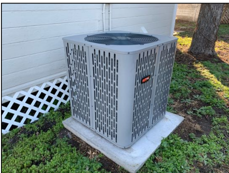
Trane condensing unit at back exterior
