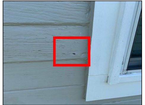
Wood siding decay/rot at the right side of the home
