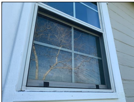
Kitchen window fogged
