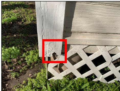
Wood trim decay/rot at the left side of the home
