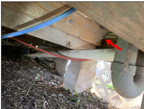
Floor joist decay/rot below laundry room
