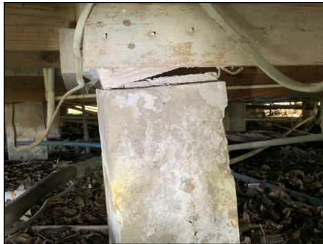
Piers/blocks damaged/leaning inadequately supporting
