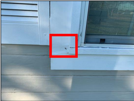
Wood trim decay/rot at the front of the home
