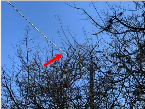
Overhead electrical service inadequate tree clearance
