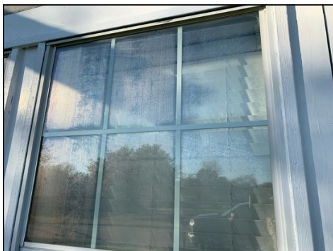
Living room window fogged
