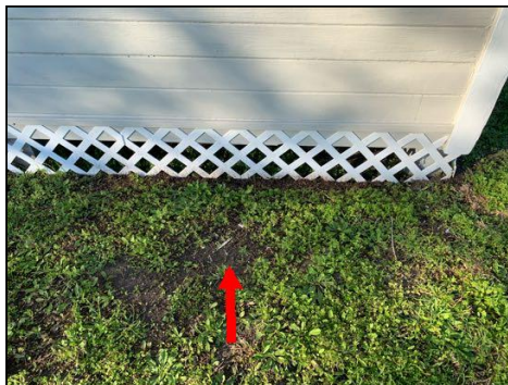
Grade slopes toward the crawlspace at the front of the home
