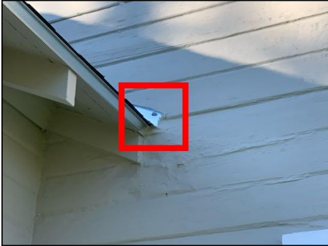
No kick out/diverter flashing at the front of the home
