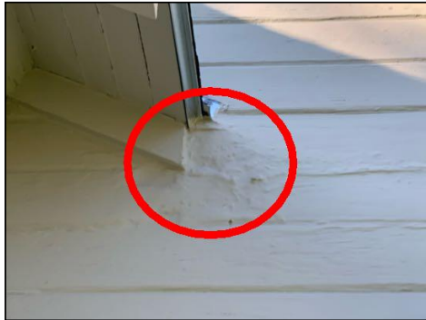
Wood siding decay/rot at the front of the home
