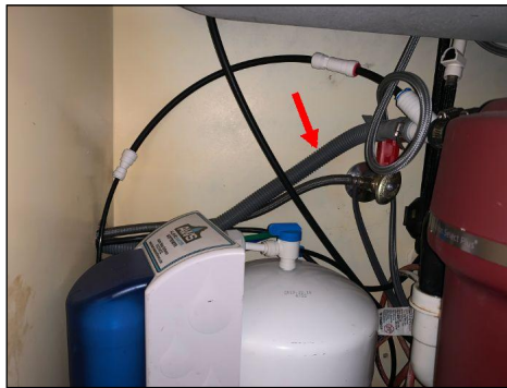
No high loop installed in the dishwasher drain for backflow prevention
