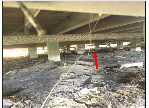
PEX Water supply plumbing in crawlspace not secured/strapped
