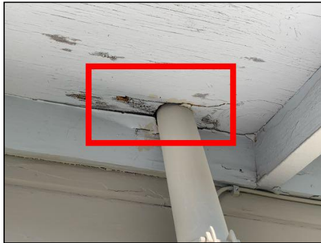
Exposed roof deck decay/rot at the left side of the home
