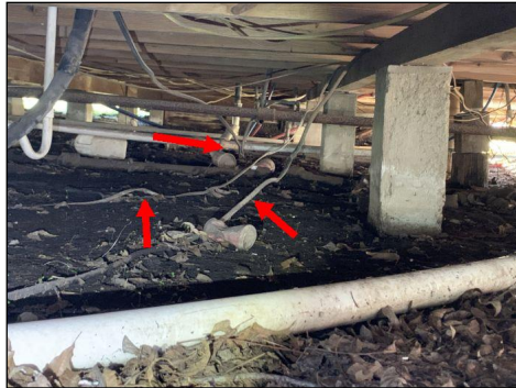
Unsecured electrical wiring in crawlspace beneath the home
